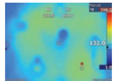
Burner Wall, Boiler #1 w/Emisshield
