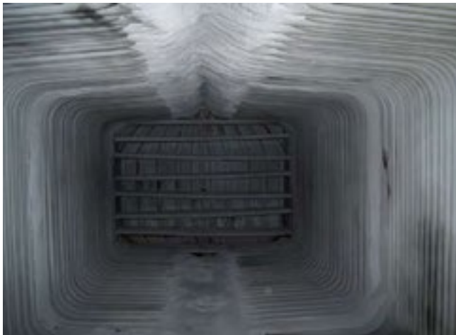
Target Wall and Tubes with Emisshield
