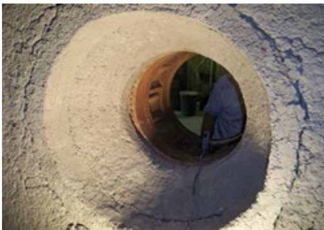
Burner Wall with Emisshield
